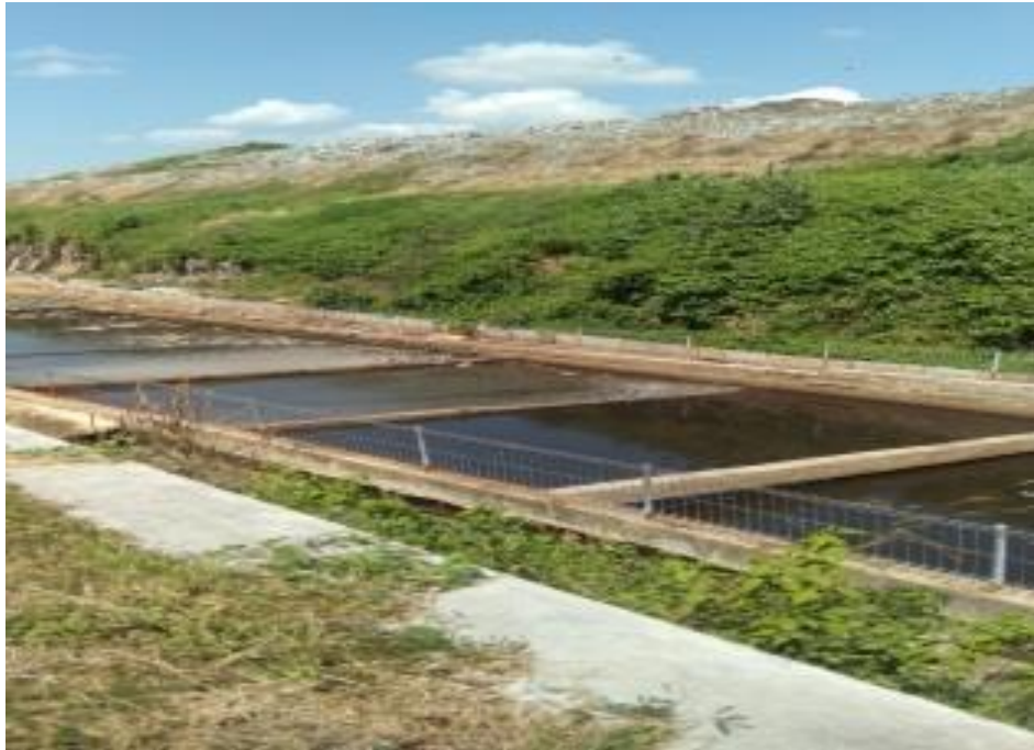
Lampiran 3 Gambar Instalasi Pengolahan Lindi
